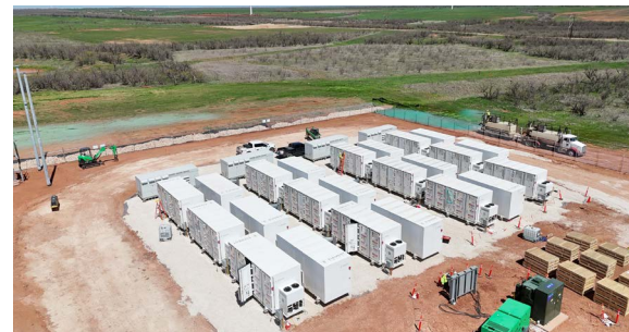
50 MWh of Reuse ESS in Texas being installed in collaboration with a North American partner
